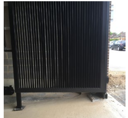
no safety edges fitted to prevent crushing
