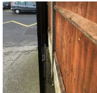
risk of gate crushing against a fence
