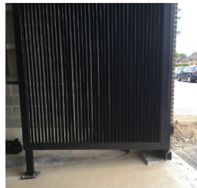
no safety edges fitted to prevent crushing
