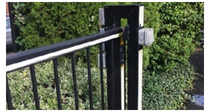
Risk of impact and crushing
