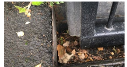
Risk of impact and crushing
