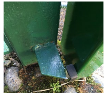
Crushing risk at ground level
