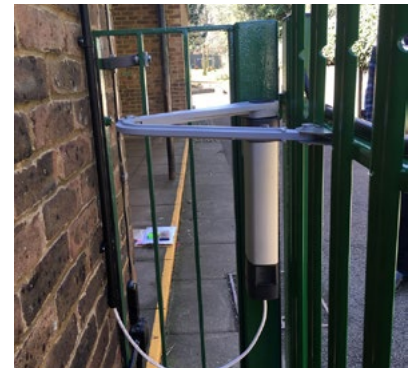
Serious crushing risk with the operator and wall
