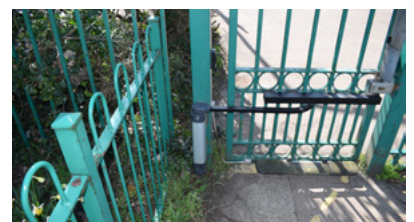
Risk of crushing
